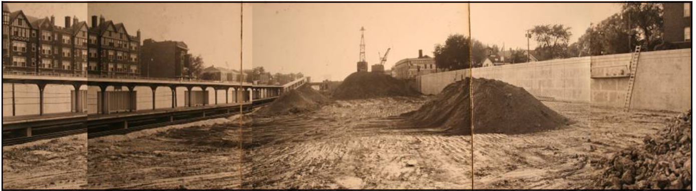
Figure 8: Construction along I-290 through Oak Park (ca 1956). Images courtesy of the Historical Society of Oak Park and River Forest
