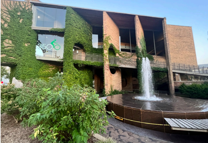
Present curtain wall enclosed balcony condition at upper level of Council Chambers .
