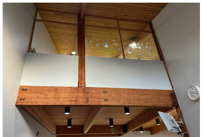
Existing conditions at Kitchen/Lounge area on the First Floor looking toward Mezzanine.
