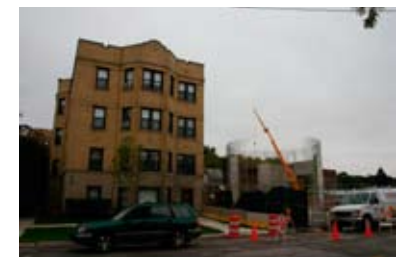
Figure 5.12: A new Oak Park public works facility is now under construction on South Boulevard.
