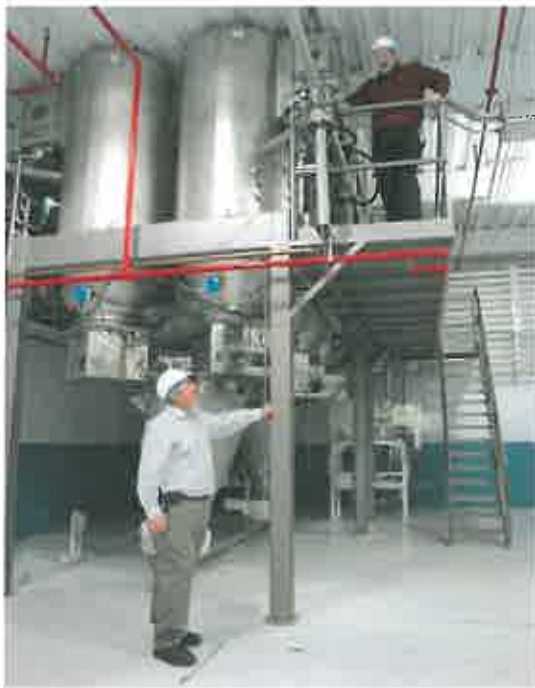
▲ Jeff Kozloski (below), plant engineer, and Jeff Benry, sanitation manager, examine conditions among bins composing the minor ingredients storage system.
