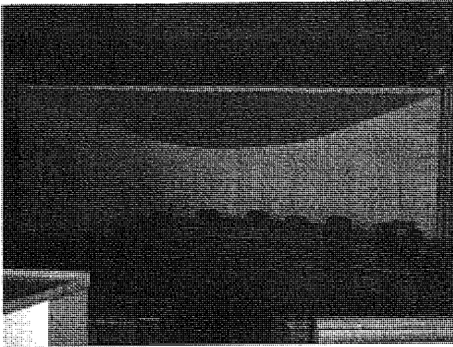
Council Chambers –the supply air is above the gyp board ceiling
