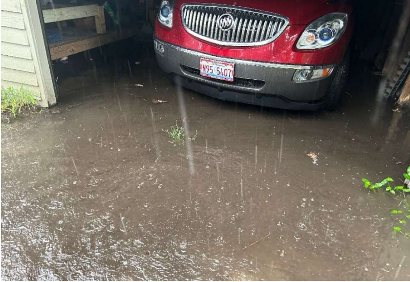
Water pools in south garage with rain/snow, and has caused rotting wood and structure damage.
