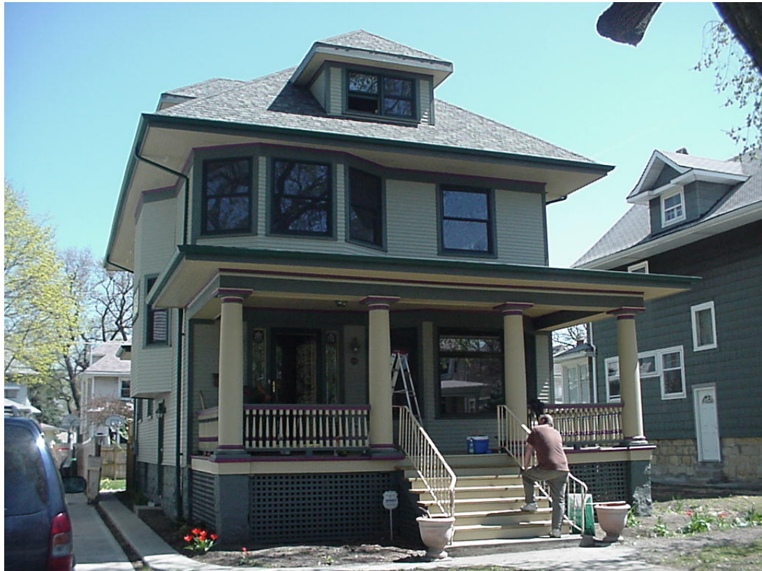
808 S. Elmwood Avenue (FIRE RESTORATION) S. T. Gunderson & Sons, 1908 Nick and Deanne Alexander Emergency Restoration Services
