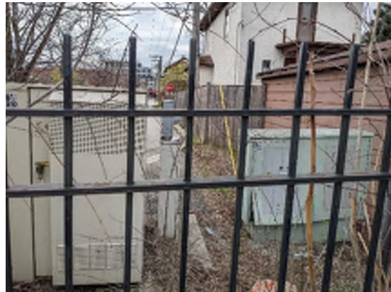
Southeast corner of property, transformers
