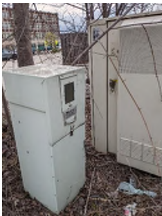
Southeast corner of property, transformers
