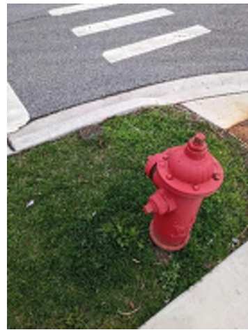
Northwest corner of property, water access and hydrant
