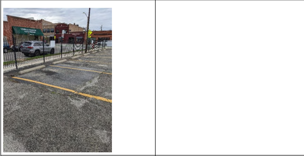
Western edge of property, pavement patch
