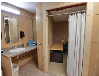
Poor layout at vanity within women's locker room
