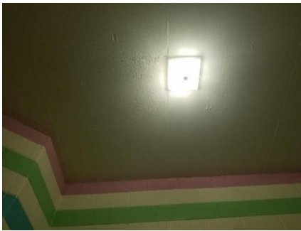
Typical detention cell lighting fixtures
