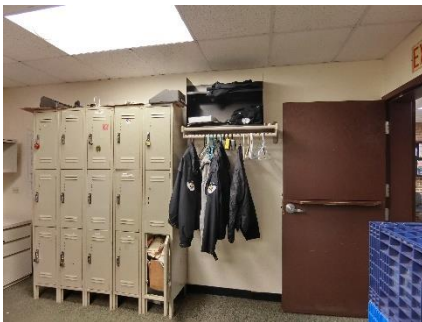
Non-compliant fire rated Dutch door at Parking Enforcement
