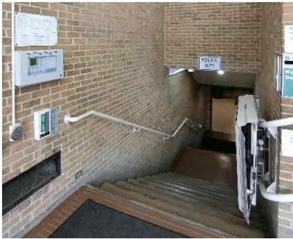
Non-functioning ADA chair lift
