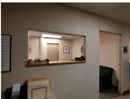
Non-ADA compliant service window
