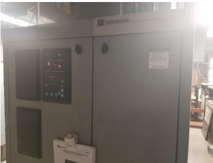
Main emergency transfer switch
