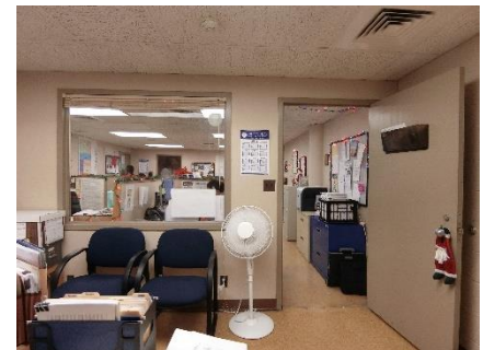
Insufficient air circulation
