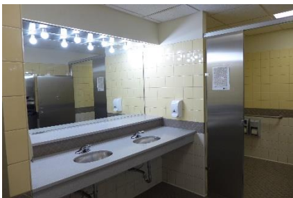
Recently updated plumbing fixture
