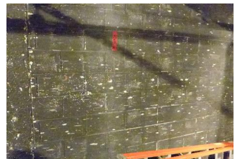
Unprotected CMU walls in Firing Range
