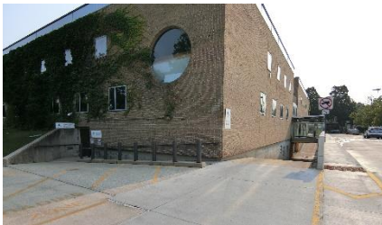
Non-compliant ADA ramp
