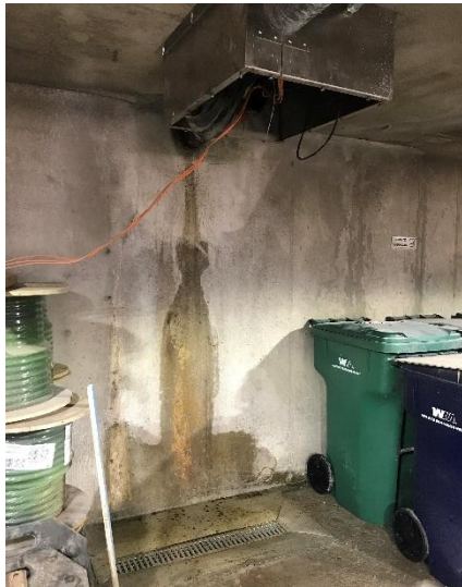
Water infiltration at pipe penetration
