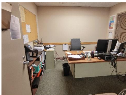
Extension cords laying on floor due to insufficient electrical outlets
