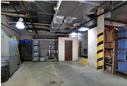
No ADA access to Sally Port
