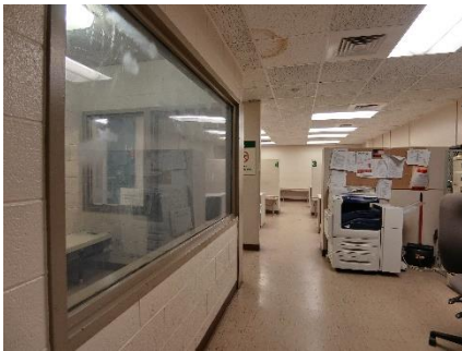
Security Glazing on lock up cell is damaged and cloudy
