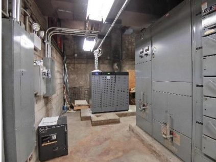
Main electrical room
