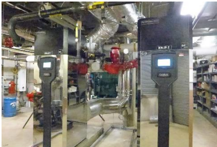
Existing boilers recently replaced
