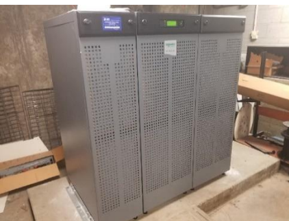
UPS battery back-up system
