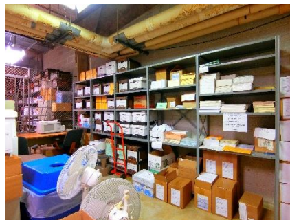
Water damaged pipes above record storage
