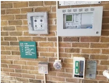
Fire alarm annunciation panel
