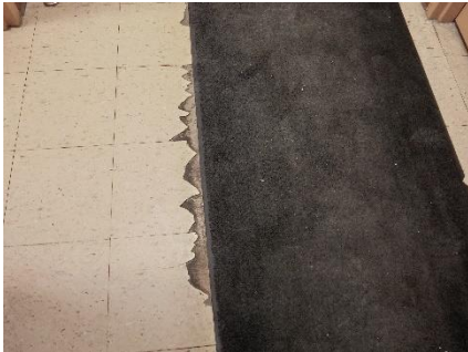
Chipped flooring outside conference room
