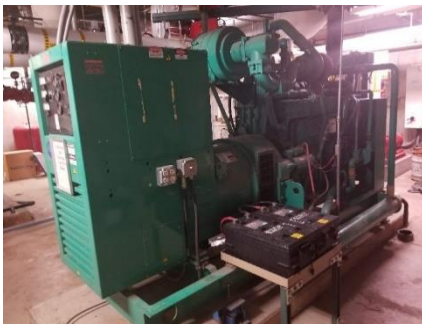
Main gas-fired back-up generator set
