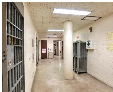
Damaged ceiling tiles within detention area
