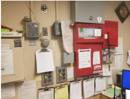
Fire alarm main control panel
