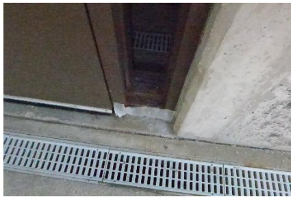
Steel door frame is corroding
