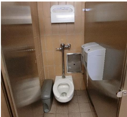
Inaccessible toilets in locker rooms
