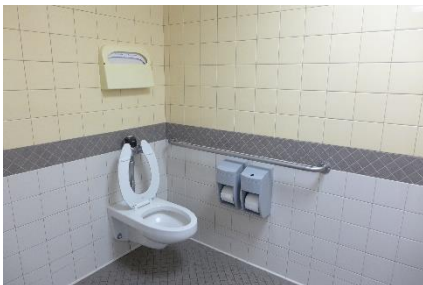
Non-compliant ADA grab bars
