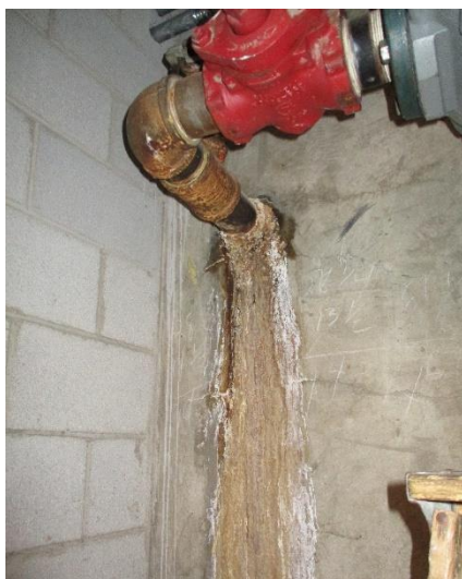
Water infiltration and corrosion at pipe in mechanical room
