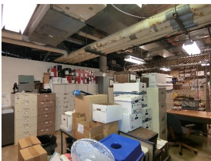
Non-compliant fire rated wall at record storage.
