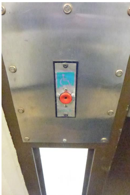
Damaged buttons at elevator
