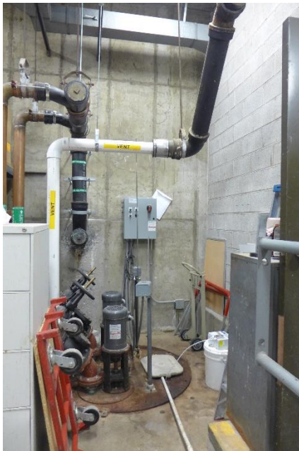
Existing ejector and sump pumps
