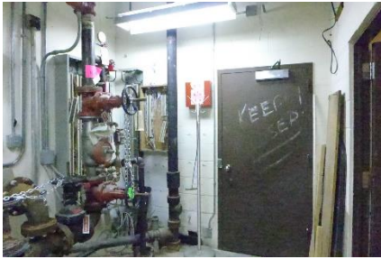
Unsecured door leading to detention area
