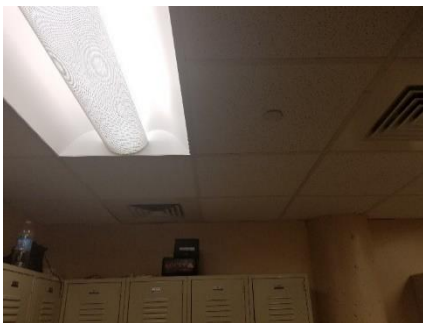
Typical updated indirect lighting fixtures
