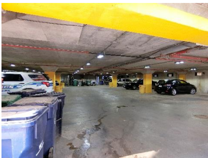
Steep slope and low head clearance at parking garage
