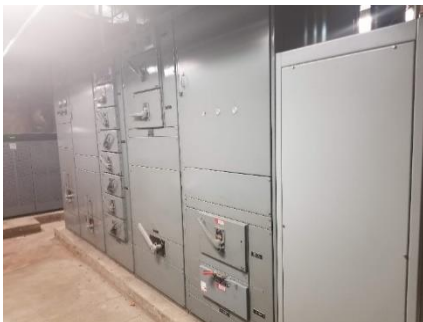
Main electric service switchboard
