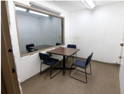
Damaged acoustical walls within interview rooms
