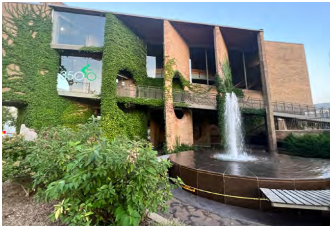
Present curtain wall enclosed balcony condition at upper level of Council Chambers .
