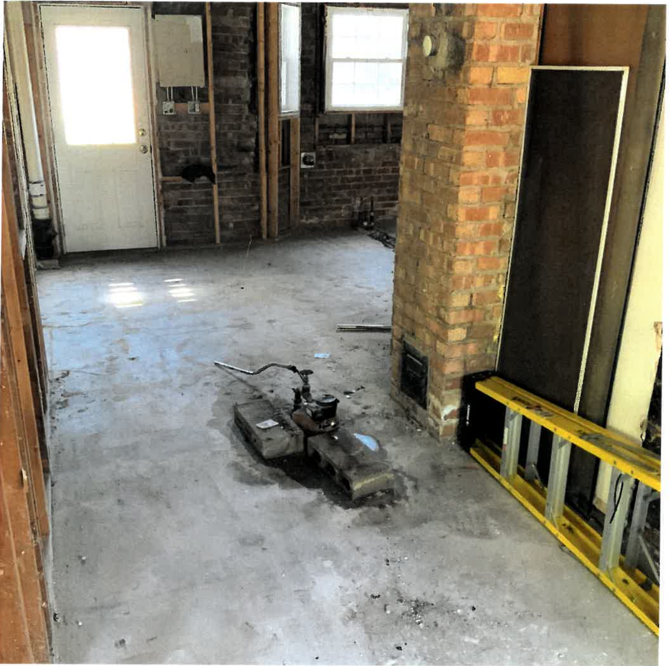
Looking from the front door toward the back, the water service comes up directly in the middle of the home. The flue and chimney for the furnace and water heater can be seen immediately to the right in the photograph above.
