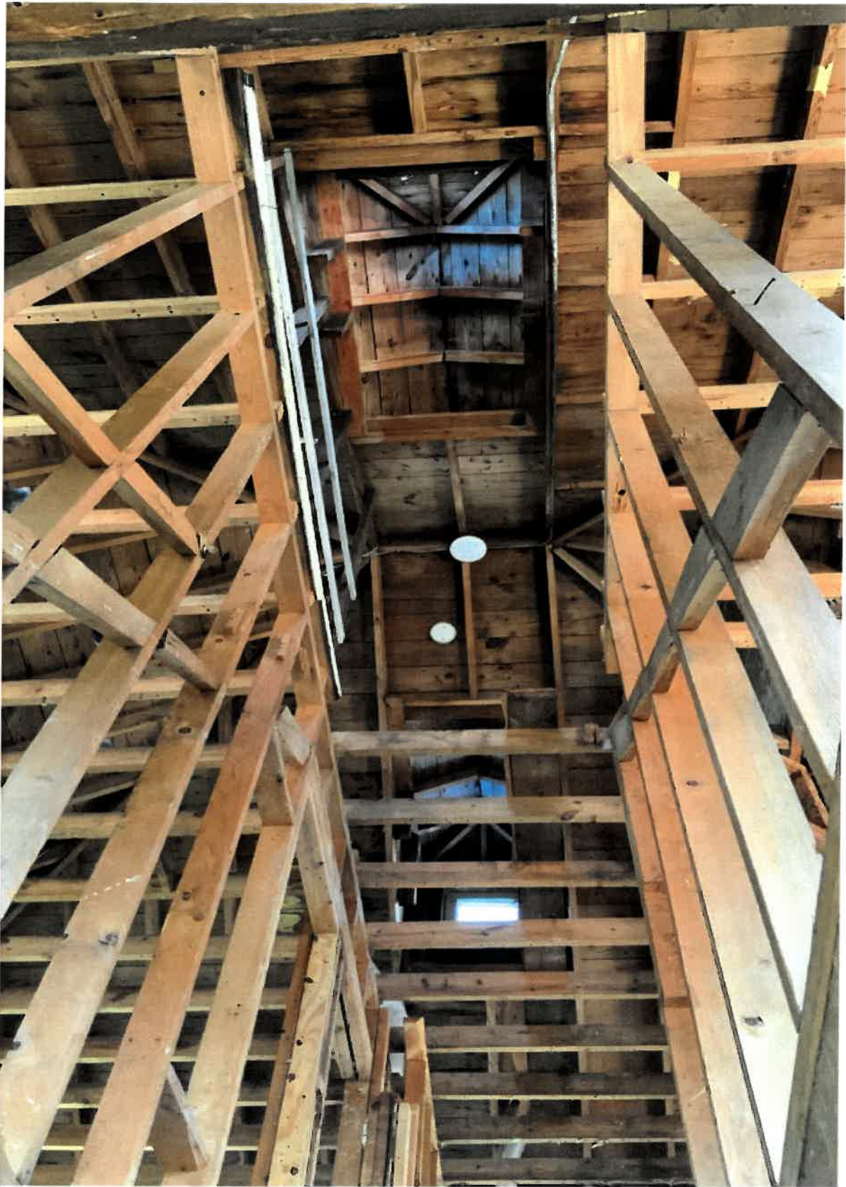
Looking up through the old stairwell toward the second floor and on up to the attic and roof rafters above. The home has been fully striped of all finishes, electrical, plumbing and HVAC. All that remains is the bare structure.
