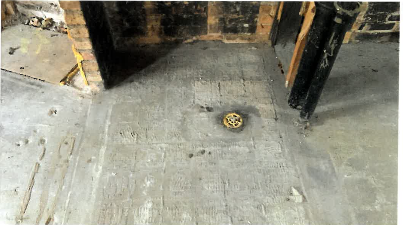
This is the location of the first floor bathroom. Note the hub for the toilet and count the number of 6" tiles that documents the actual width of the space. 6 \text{ tiles} \times 6" = 36" overall width.
