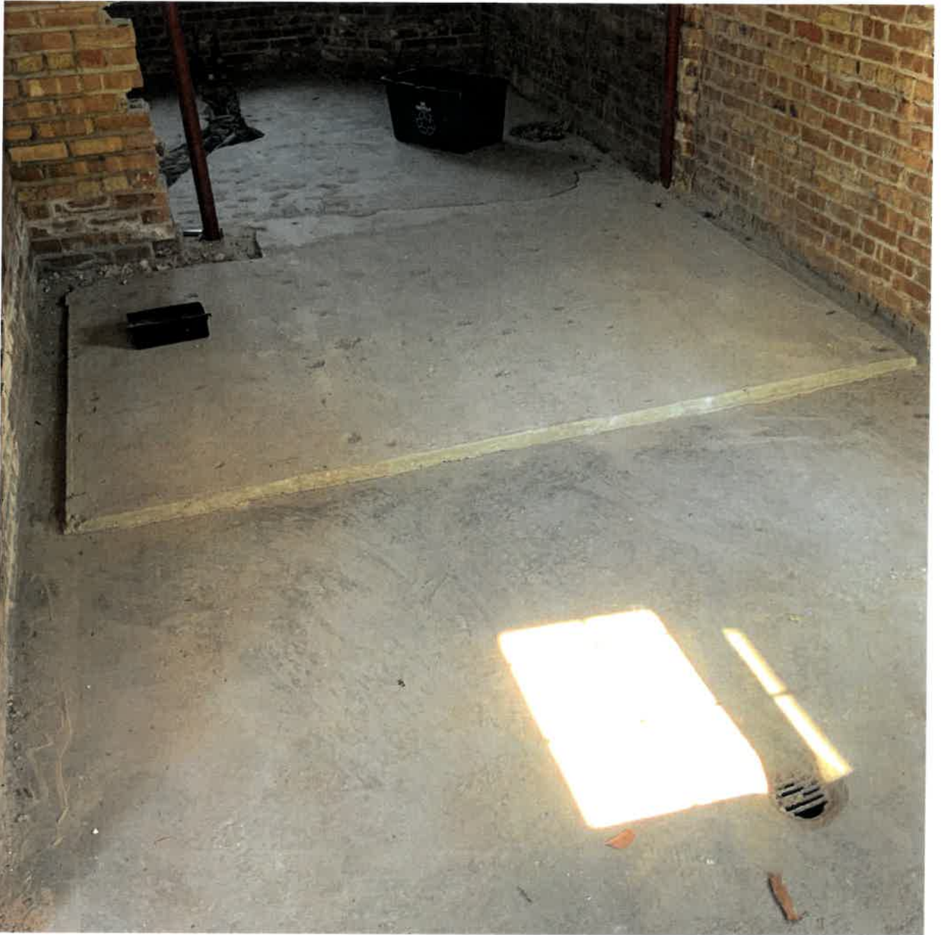
Within the garage bay, the floor has been partially leveled. Note the floor drain that also needs to be capped and closed off.
