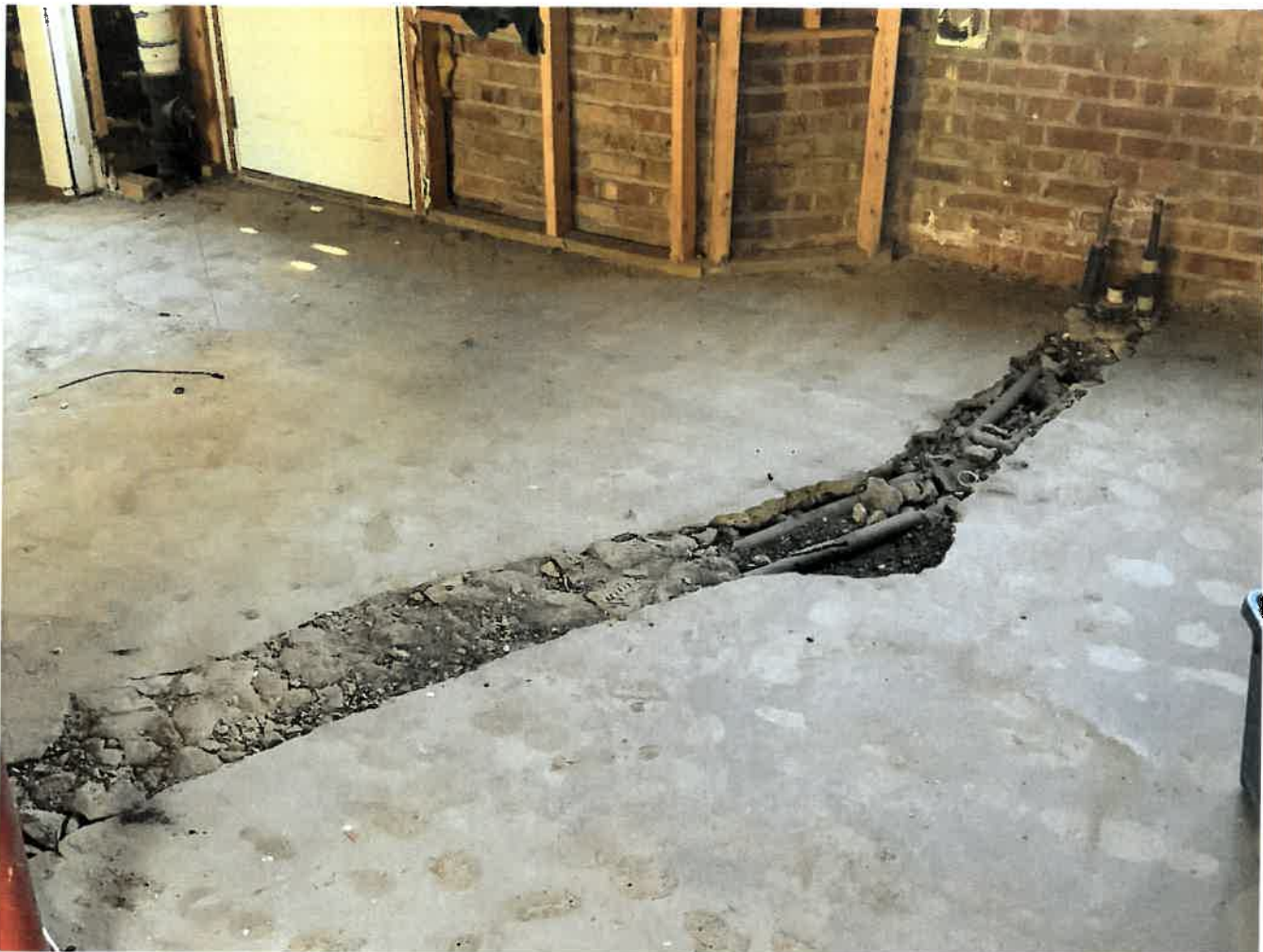
The existing floor has been opened to access the piping below the floor line. This will of course need to be repaired.
