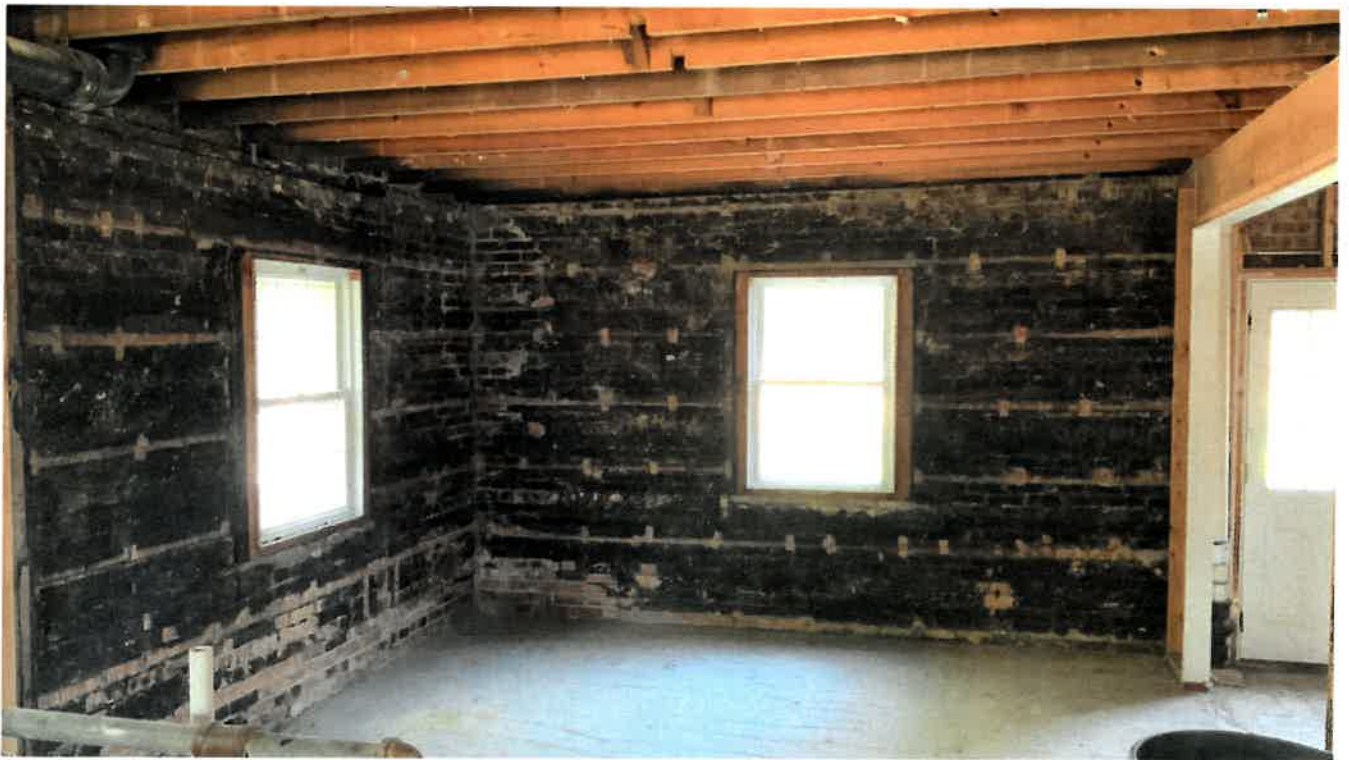
Looking toward the north east corner of the building interior. Notice the joists with the notches cut directly in the middle of the span. The joists will have to removed and replaced.
