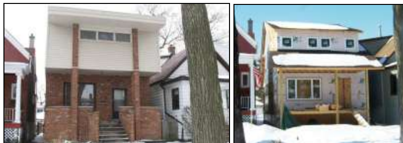
835 N. Lombard was destroyed in a fire, and the new house is under construction
