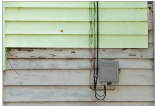
In some cases, removing non-historic siding like the aluminum pictured above may reveal historic wood siding underneath that is in good condition.
