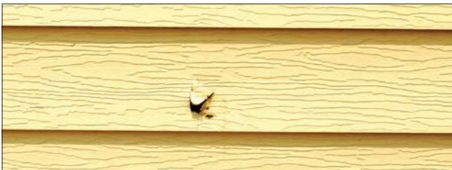
Repair of this puncture requires replacement. Replacement of this aluminum siding is the best way to repair this puncture. A wood-grained texture is generally inappropriate.
