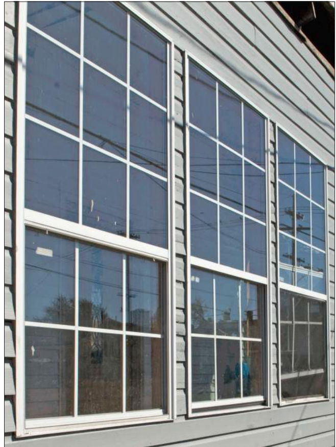
The 9/6 vinyl replacement windows in the image have applied muntins, are mounted flush against the outside wall, and lack the depth of traditional windows. They do not have trim or casings including a drip cap and sill. As a result they are inappropriate and diminish the historic character of the building.
