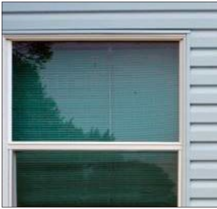
The window frame pictured has been completely covered with vinyl siding. The articulation formerly provided by the frame has been replaced with a J-channel for the vinyl siding. Without the frame, the visual dimensions of the window are changed and character of the building is diminished.
