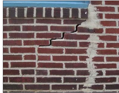
A previous vertical crack has been improperly repaired with hard grout smeared onto the wall surface. The second diagonal crack suggests a settlement or foundation problem.
