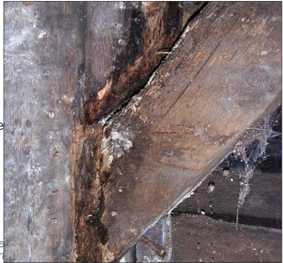
The dark areas at the top and side of the diagonal wood brace indicate moisture. The end of the diagonal wood frame is rotting. The cause of the moisture infiltration should be addressed, and the wood framing repaired or replaced.
