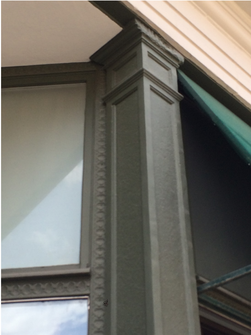
Photo 8: Detail of existing transoms and awning. Note the missing column capital trim that is proposed for restoration.
