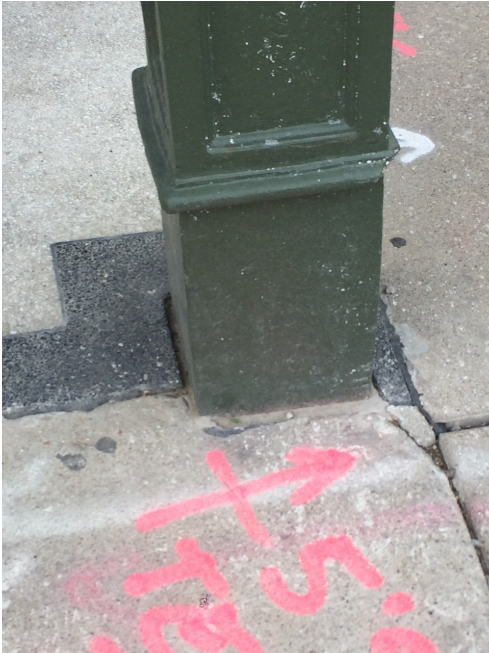
Photo 9: Detail of the corner columns showing the missing base. The base will be restored as part of the project.
