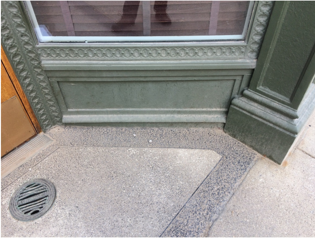
Photo 7: Detail of the recessed entry bulkhead and decorative trim. The bulkhead details will be matched; the decorative trim will be reused.
