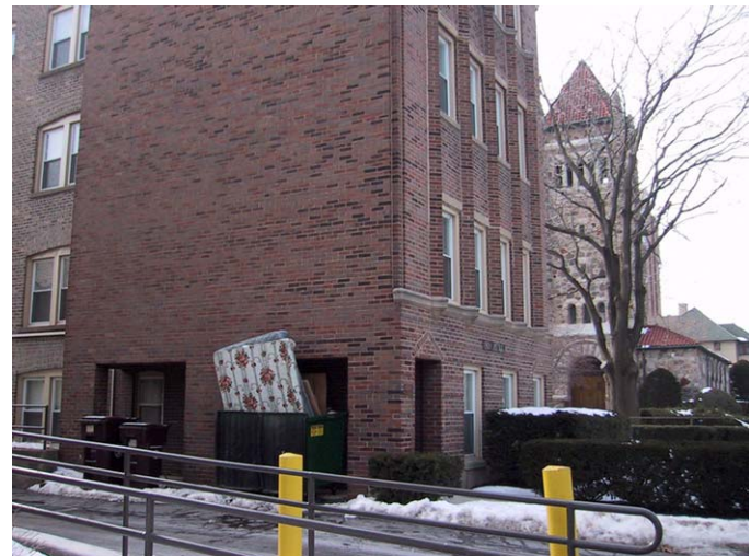
Inappropriate Trash Screening
