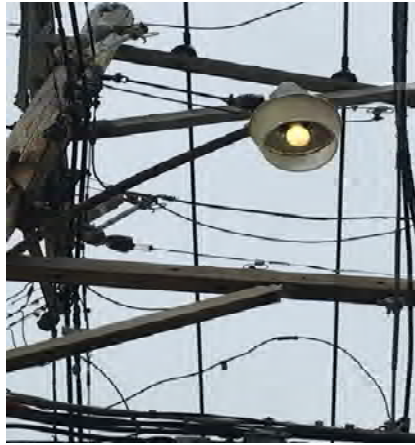
100W Mercury Vapor Alley Light Fixture
