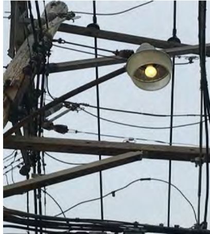
100W Mercury Vapor Alley Light Fixture
