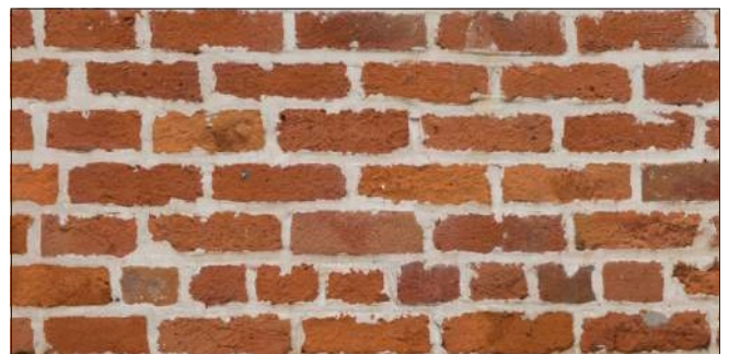
The surface of the brick has been damaged by inappropriate cleaning methods. A power tool was likely used to cut-out joints prior to repointing, resulting in the over-cut vertical joints.
