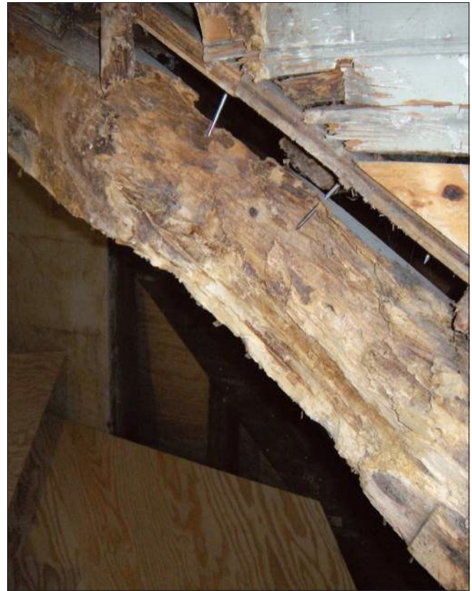
The surface of this roof rafter has rotted and is no longer capable of holding the nails from the plywood sheathing. This rafter is rotted and beyond its useful life. It should be replaced.
