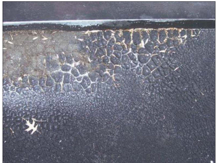
The “alligatored” roof surface shown here indicates deterioration and possible need for replacement.
