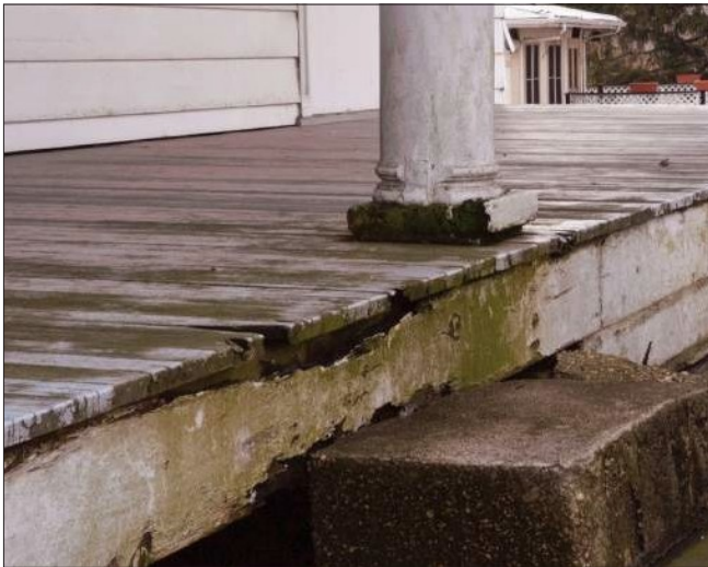
Porches, steps, and other areas where the woodwork is laid horizontally or located close to the ground are often first to deteriorate. Ongoing exposure to moisture can lead to rot of the column bases, porch deck, and apron.
