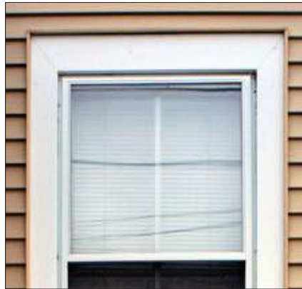
Aluminum capping has been installed over the window frame. Aluminum capping usually lacks the profile and detail of wood trim. It can also trap moisture within the wall surface that can accelerate rot and deterioration.
