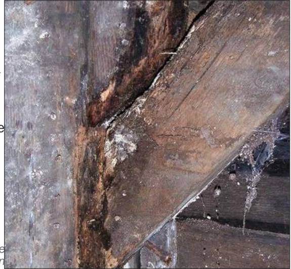
The dark areas at the top and side of the diagonal wood brace indicate moisture. The end of the diagonal wood frame is rotting. The cause of the moisture infiltration should be addressed, and the wood framing repaired or replaced.
