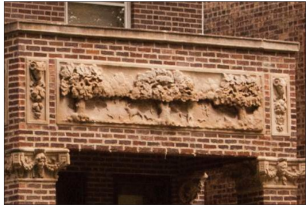
The highly detailed, deep decorative relief in the panels and the capitals of the porch piers are made from terra cotta. A variety of terra cotta patterns and shapes were available at the beginning of the 20th century, providing a relatively inexpensive means of “decorating” building surfaces.
