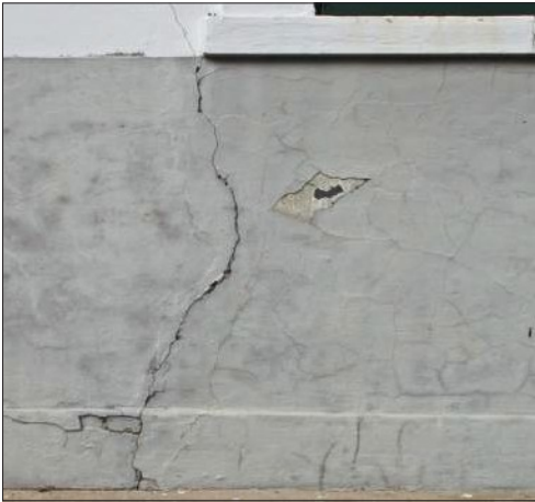
The crack from the window sill shown here might be a sign of building settlement. Review wall for other signs of movement. Repair crack and apply a lime-based paint for a uniform appearance.
