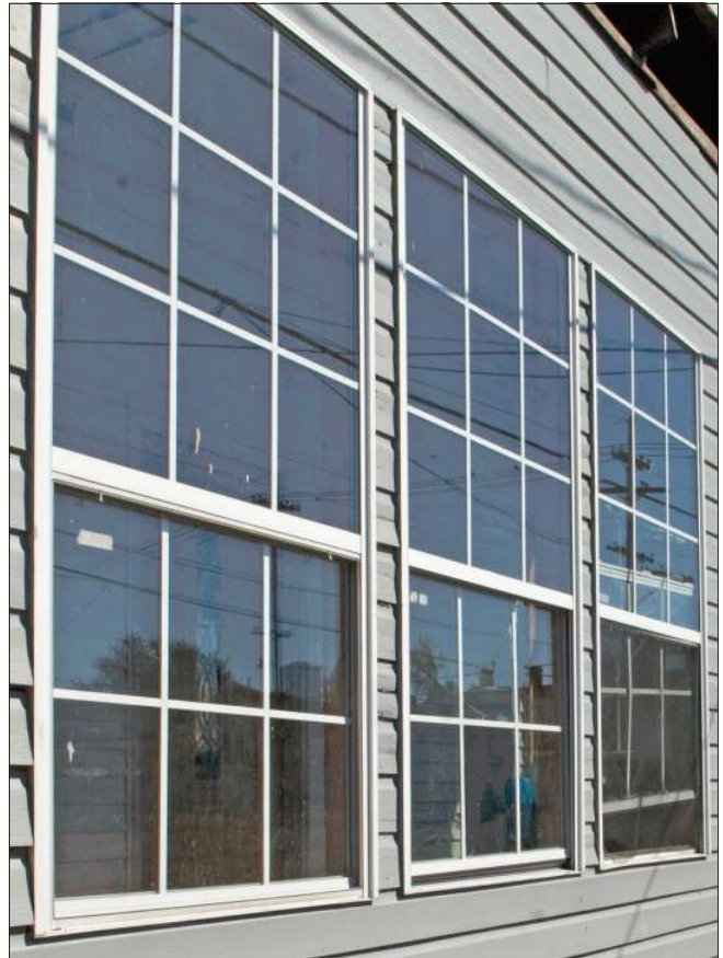
The 9/6 vinyl replacement windows in the image have applied muntins, are mounted flush against the outside wall, and lack the depth of traditional windows. They do not have trim or casings including a drip cap and sill. As a result they are inappropriate and diminish the historic character of the building.
