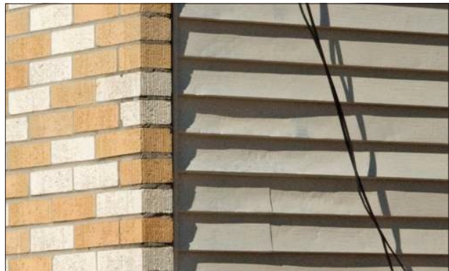
The left wall of this wood-framed house has been covered with brick veneer. The addition to the right has been covered with vinyl siding. Both are inappropriate materials and should not be used on historic buildings.
