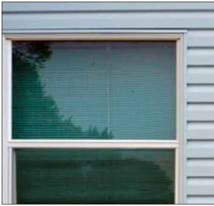
The window frame pictured has been completely covered with vinyl siding. The articulation formerly provided by the frame has been replaced with a J-channel for the vinyl siding. Without the frame, the visual dimensions of the window are changed and character of the building is diminished.
