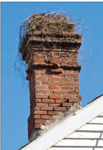
This chimney is leaning and has visible open joints. The chimney should be dismantled and rebuilt to match the existing form and details.
