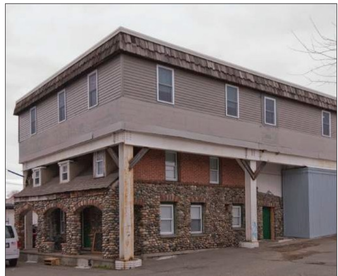
This 3rd floor addition overwhelms the historic building and is inappropriate. Its scale is substantially larger, the side gable roof form has been altered to a flat roof, the footprint has been greatly expanded, the window size and proportions are dramatically different, and trim, details, and materials vary greatly from the historic building.
