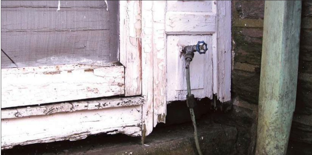
In this photo, the wood base is in contact with the concrete step. Regular wood dampness can eventually lead to rot and deterioration. The spigot should be checked for leaking and the downspout checked to make sure there is appropriate drainage away from the building foundation.
