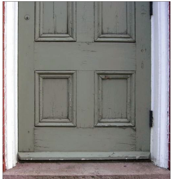
Wood checking and peeling paint is visible. Minor repair and maintenance can prolong the serviceable life of this door. The trim at the bottom rail of the door helps prevent storm water from entering the building.
