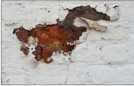
The paint here is likely peeling because it is incompatible with the brick and moisture was trapped in the wall. The paint should be removed and moisture problems addressed.
