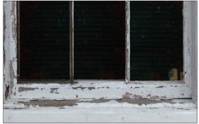
Typically, the deterioration of wood windows first occurs at the sill. Peeling paint can allow moisture to enter wood and cause rot. Regular repainting is recommended to provide a protective barrier against moisture.
