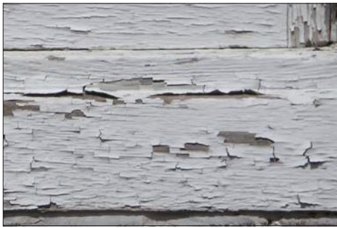
The window sill and jamb have peeling paint and some checking or splitting. Removal of the loose paint will allow the wood to be inspected for signs of rot.
