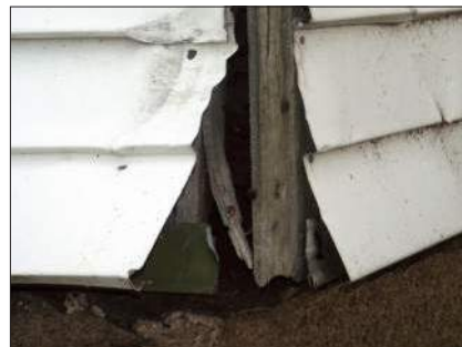
Aluminum and vinyl siding were sometimes installed to conceal an underlying problem. In some cases, removal might be necessary to repair a deteriorated condition.
