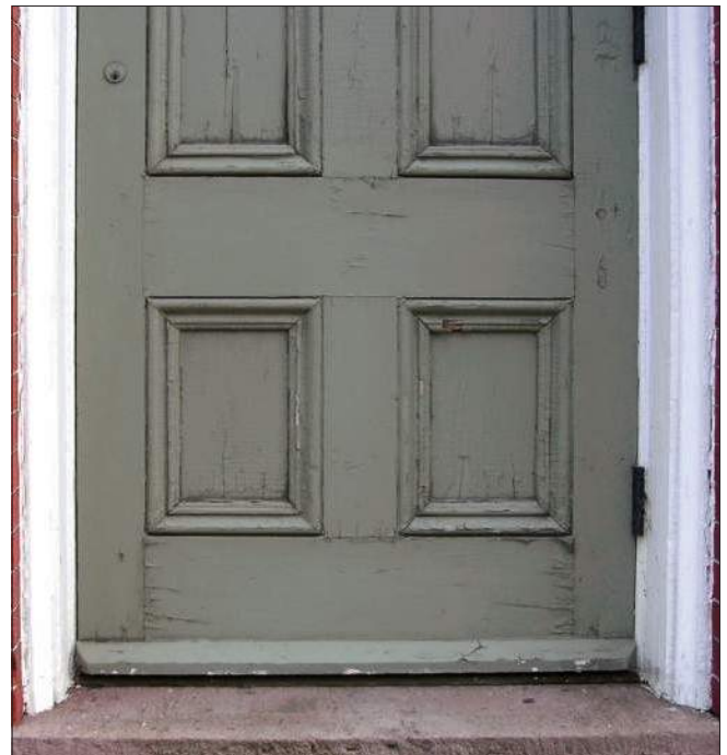
Wood checking and peeling paint is visible. Minor repair and maintenance can prolong the serviceable life of this door. The trim at the bottom rail of the door helps prevent storm water from entering the building.
