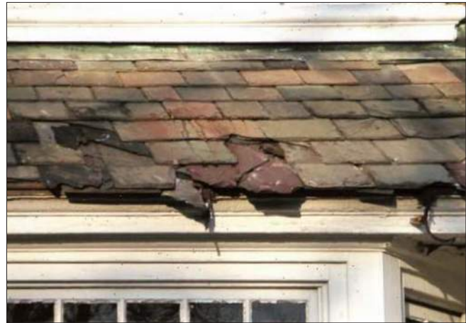
In the above photo, slates are cracked, dislodged, and missing. Some of the surfaces are flaking and approximately 25- 30% of the slates on this roof are either missing or damaged. Given the extent of the problems, roof replacement would be appropriate.
