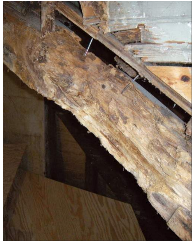
The surface of this roof rafter has rotted and is no longer capable of holding the nails from the plywood sheathing. This rafter is rotted and beyond its useful life. It should be replaced.
