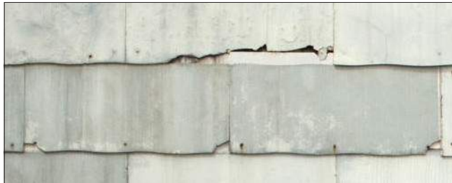
Asbestos siding is often embossed with a wood grain pattern. The removal of asbestos siding can be dangerous and should be undertaken by trained professionals.
