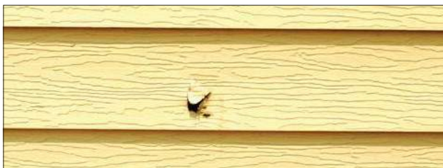
Repair of this puncture requires replacement. Replacement of this aluminum siding is the best way to repair this puncture. A wood-grained texture is generally inappropriate.
