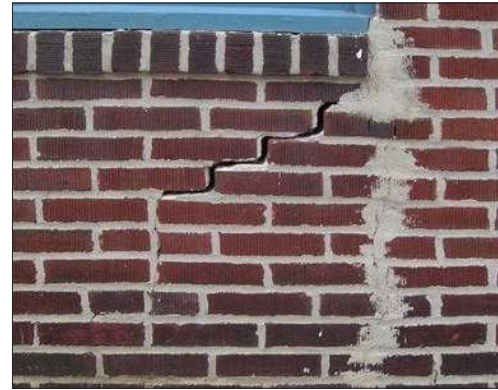
A previous vertical crack has been improperly repaired with hard grout smeared onto the wall surface. The second diagonal crack suggests a settlement or foundation problem.
