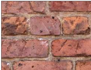
19th Century Brick - A soft, fired-clay, fairly regularly shaped building component, often with color and surface variations.
