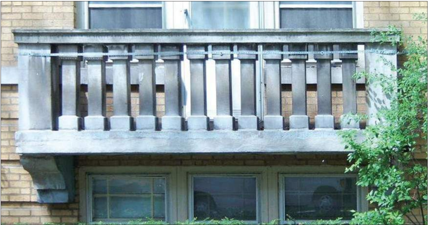
This limestone balcony is supported by brackets flanking the window below and is accessed by a central door. The railing is comprised of square balusters with corner piers.
