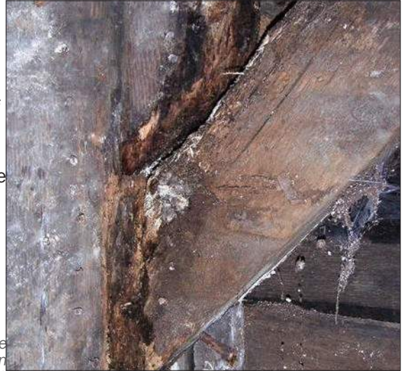
The dark areas at the top and side of the diagonal wood brace indicate moisture. The end of the diagonal wood frame is rotting. The cause of the moisture infiltration should be addressed, and the wood framing repaired or replaced.
