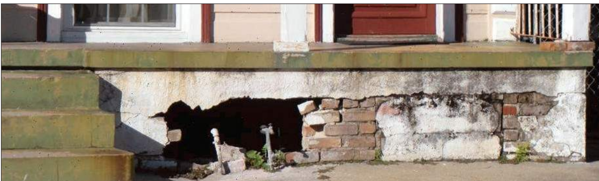
The stucco has not been maintained and the bricks under the porch post are falling out of position. The dislodged bricks can lead to structural problems at the porch if not repaired.
