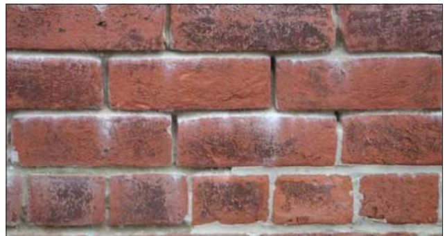
The mortar, particularly in the vertical joints, is deteriorated, increasing the potential for water infiltration. The area in the lower right of the photograph was repointed and mortar was smeared over the surface of the brick rather than tooled. Replacement mortar should match the historic in appearance, color, texture, hardness, and joint profile.
