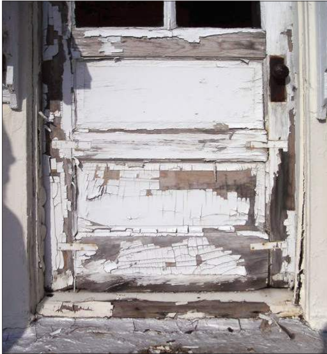
The paint on this door has alligatored, and severe cracking is visible. The paint should be removed down to bare wood and the door properly repaired prior to repainting.
