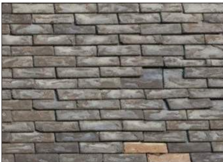
Individual missing or damaged slates can often be replaced, extending the serviceable life of the roof and postponing costly replacement.
