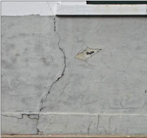
The crack from the window sill shown here might be a sign of building settlement. Review wall for other signs of movement. Repair crack and apply a lime-based paint for a uniform appearance.
