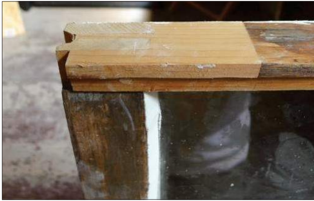
One of the advantages of historic wood windows over modern prefabricated units is reparability. This photo demonstrates a dutchman repair at the corner of a historic wood window. Also note the new glazing putty.
