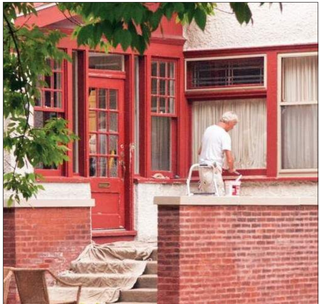
Proper preparation before repainting, including hand scraping, sanding and washing, as well as using quality paint and primer appropriate for the material, will result in a better-quality job. The tarp in the photograph does not meet current EPA requirements for protection of the soil and environment.
