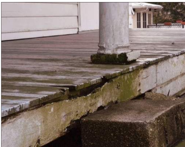
Porches, steps, and other areas where the woodwork is laid horizontally or located close to the ground are often first to deteriorate. Ongoing exposure to moisture can lead to rot of the column bases, porch deck, and apron.
