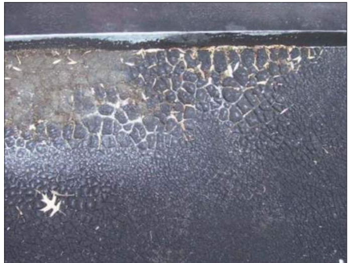
The “alligatored” roof surface shown here indicates deterioration and possible need for replacement.
