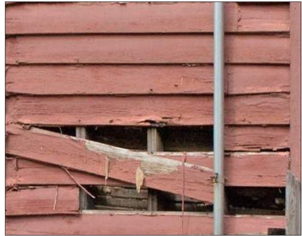
Gaps or openings in wood siding should be repaired to prevent moisture and pests from entering the wall cavity.
