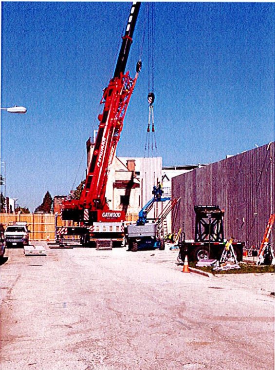
Precast wall panel being set in place at west end of substation, 06-06-14.
