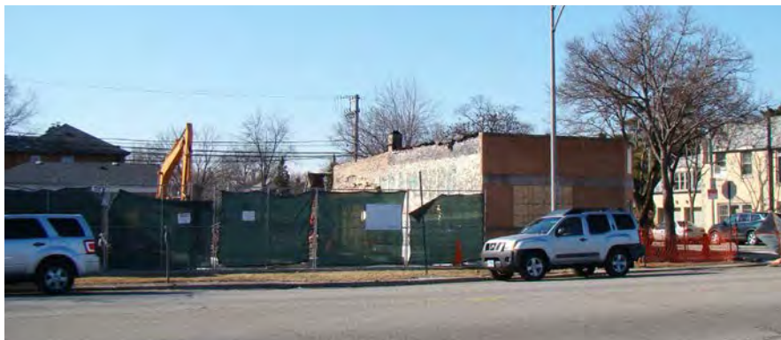
New residential construction is underway at the east corner of North and East Avenues.
