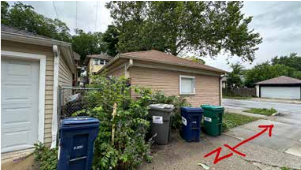
Photo 11. View of Existing 1150 S.Cuyler's garage East Side from alley facing North West.
