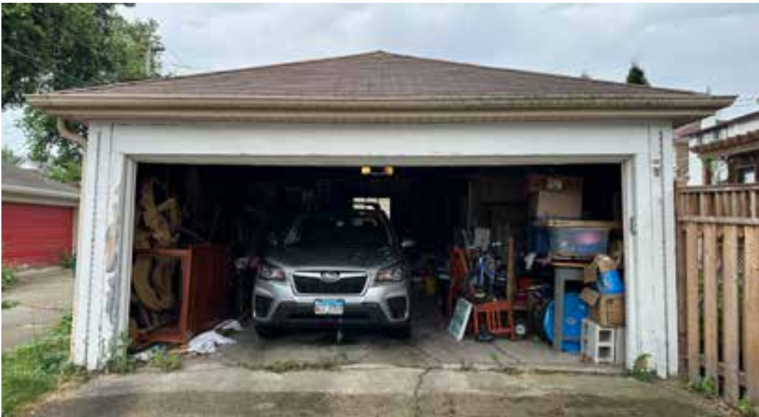
Photo 4. North Side of Garage (1150 S.Cuyler) with existing Garage Door opening onto Filmore Ave. Facing South
