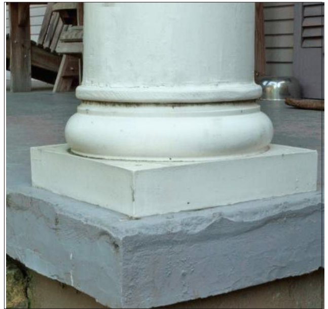
The porch column above is wood but the base has been replaced with a composite material that is visually similar to the former wood base.
