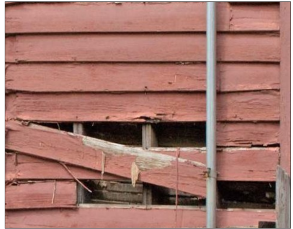
Gaps or openings in wood siding should be repaired to prevent moisture and pests from entering the wall cavity.
