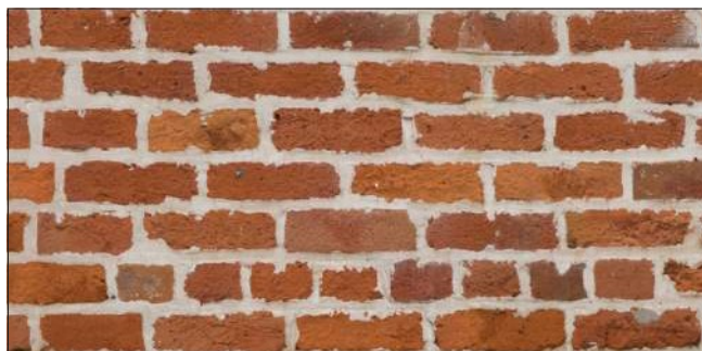
The surface of the brick has been damaged by inappropriate cleaning methods. A power tool was likely used to cut-out joints prior to repointing, resulting in the over-cut vertical joints.
