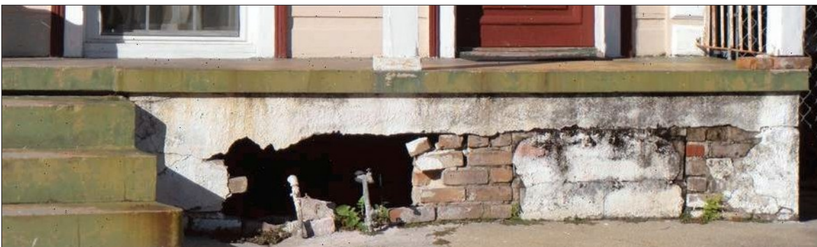
The stucco has not been maintained and the bricks under the porch post are falling out of position. The dislodged bricks can lead to structural problems at the porch if not repaired.
