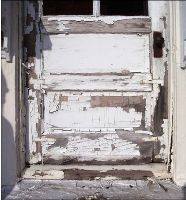
The paint on this door has alligatored, and severe cracking is visible. The paint should be removed down to bare wood and the door properly repaired prior to repainting.
