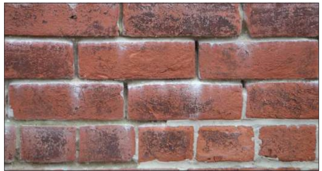
The mortar, particularly in the vertical joints, is deteriorated, increasing the potential for water infiltration. The area in the lower right of the photograph was repointed and mortar was smeared over the surface of the brick rather than tooled. Replacement mortar should match the historic in appearance, color, texture, hardness, and joint profile.
