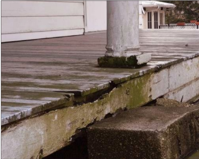
Porches, steps, and other areas where the woodwork is laid horizontally or located close to the ground are often first to deteriorate. Ongoing exposure to moisture can lead to rot of the column bases, porch deck, and apron.
