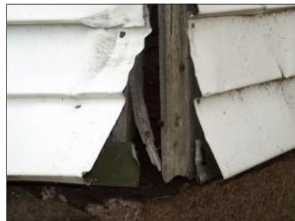
Aluminum and vinyl siding were sometimes installed to conceal an underlying problem. In some cases, removal might be necessary to repair a deteriorated condition.
