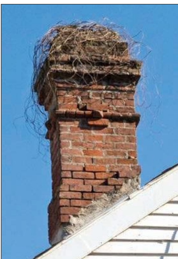
This chimney is leaning and has visible open joints. The chimney should be dismantled and rebuilt to match the existing form and details.
