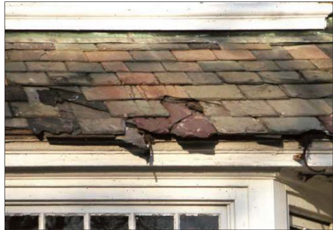
In the above photo, slates are cracked, dislodged, and missing. Some of the surfaces are flaking and approximately 25- 30% of the slates on this roof are either missing or damaged. Given the extent of the problems, roof replacement would be appropriate.
