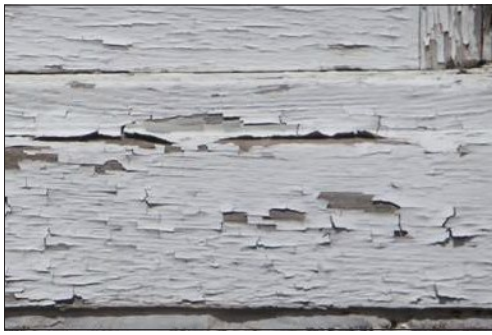
The window sill and jamb have peeling paint and some checking or splitting. Removal of the loose paint will allow the wood to be inspected for signs of rot.
