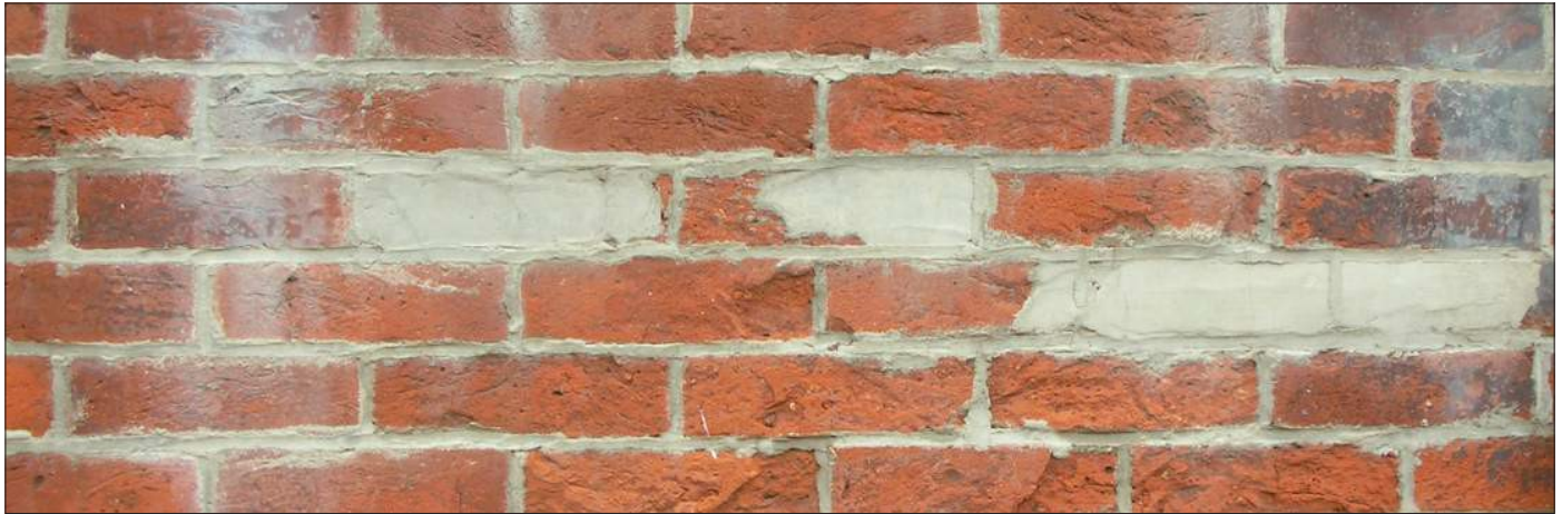
The rough texture and uneven surface of this brick suggest that an aggressive cleaning method was used. Stucco patches replace bricks and efflorescence, a powdery white substance, can be seen on the surface.
