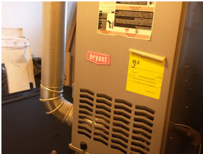
Photograph No. 13 View of the interior - second story furnace room
